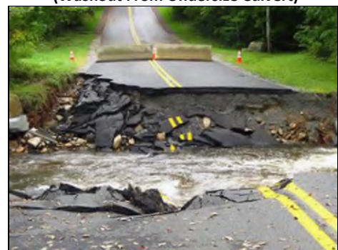
Resilience (Washout From Undersize Culvert)
