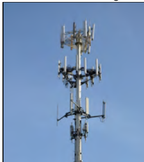
Common Tower With No Camouflage
