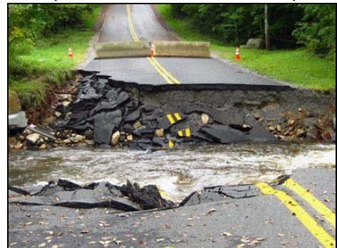
Resilience (Washout From Undersize Culvert)
